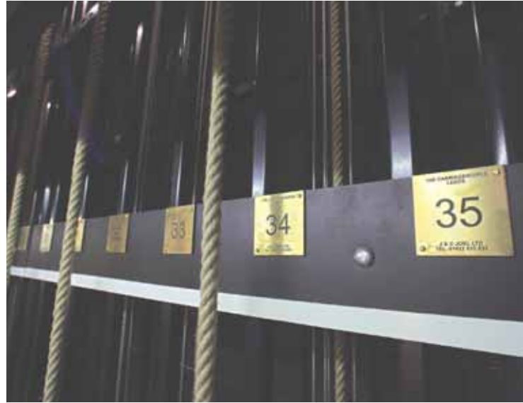
Counterweight system: Carriage Works, Leeds, UK
