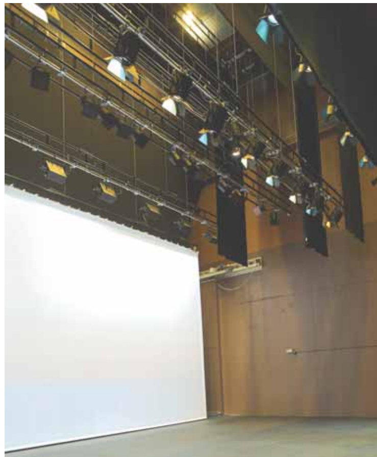
Counterweight lines and cyclorama: Solstice Arts Centre, Navan, Ireland
